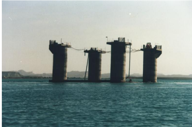
Fig.10: the caisson is located in the installation site and it is ready to be drowned
